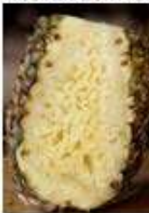
Interior soft rot
